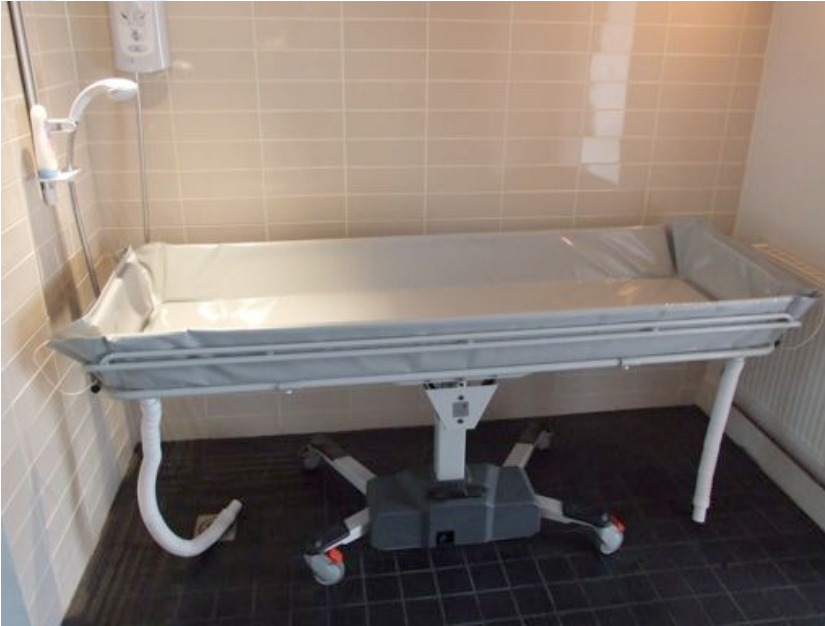
The shower trolley was small enough to fit into the recessed wet area
