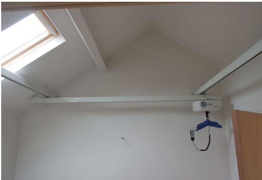
Large H system fitted on wall brackets
